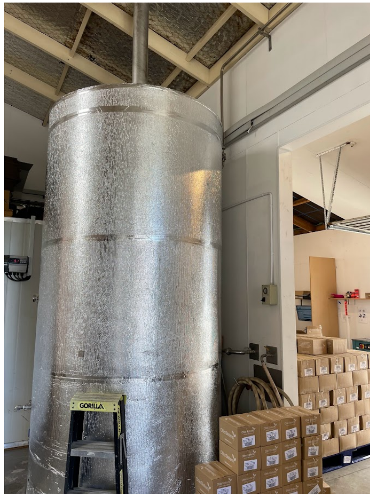
Figure 3.2: The boiler in the Chia Factory in Nelson.
