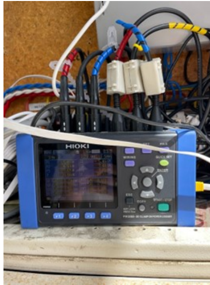
Figure 3.5: The Hioki Data logger used for monitoring.
