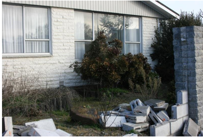
Photo 3: Non-structural damage caused by the 2011 Christchurch earthquake. (Photo taken: 03/8/2012 by Sue Chaytor)
