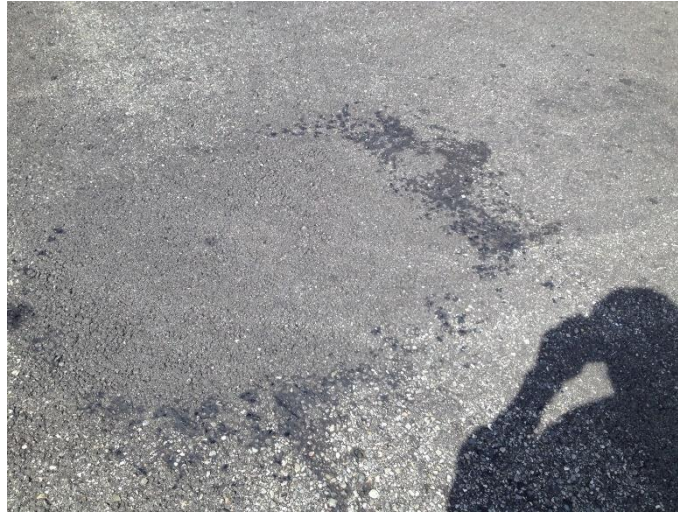
Figure 47 - Deformed area of runway requiring repeated repair
