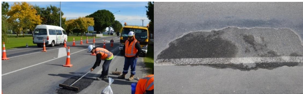
Figure 46 - Repair of site using Ultra Mender (left), and Ultra Mender repair after 4 months (right).
